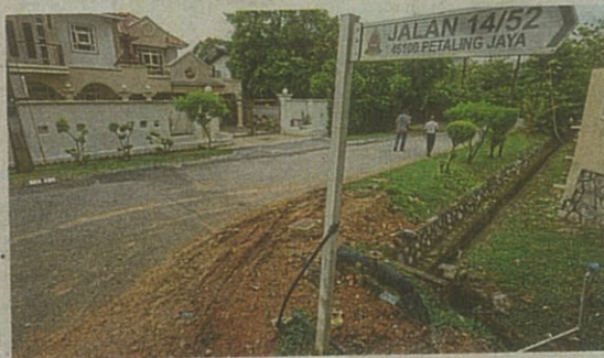
Section 14 residents say there are road depressions and sand mounds due to pipe replacement works. — GLENN GUAN/The Star
