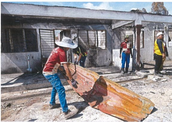
A volunteer carrying away a zinc roof sheet from a burnt house.
