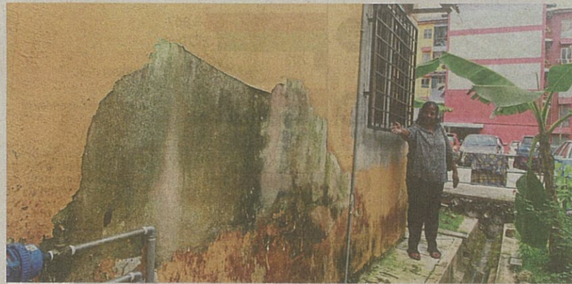
Pushpaleela says there are many cracks in Enggang Apartment (above), while residents say the overall condition of the flats, which includes Nuri Apartment (right), was poor. — Photos: KAMARUL ARIFFIN/The Star
