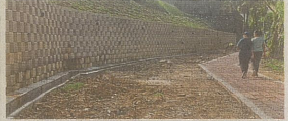
There were public complaints about the crooked retaining wall at the Astaka sports complex field in Petaling Jaya. — Filepic
