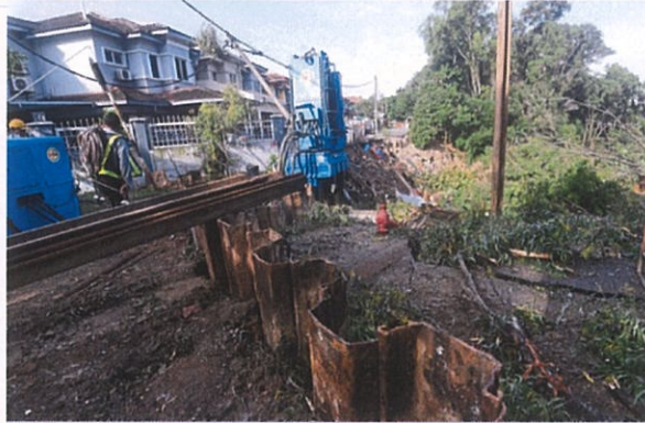
Contractors installing sheet piles to control soil movement at the site in Taman Wawasan, Puchong, after a landslide last December. — Filepic
