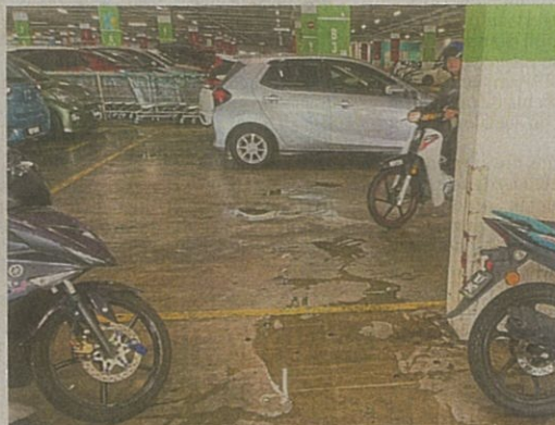
Wet floors in indoor parking lots pose risks for motorists.
