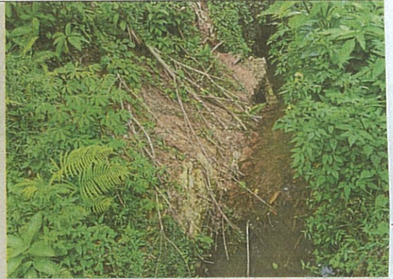
The monsoon drain along Jalan Pinggiran 3/4 is still clogged and choked with vegetation.
