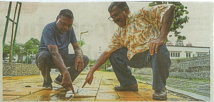
Sivam (left) and Devadass pointing at the uneven pavers. — Photos: RAJA FAISAL HISHAN/ The Star
